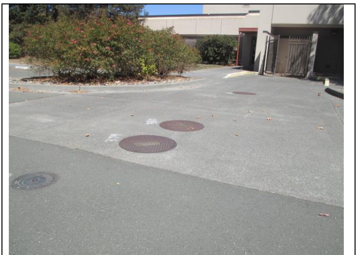
18. View of the grease interceptor system.
