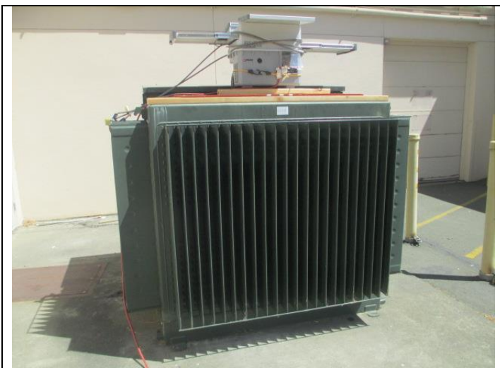
17. View of the pad-mounted transformer.
