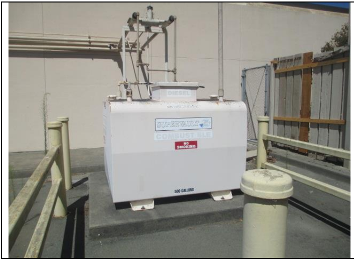
15. View of the 500-gallon diesel AST.
